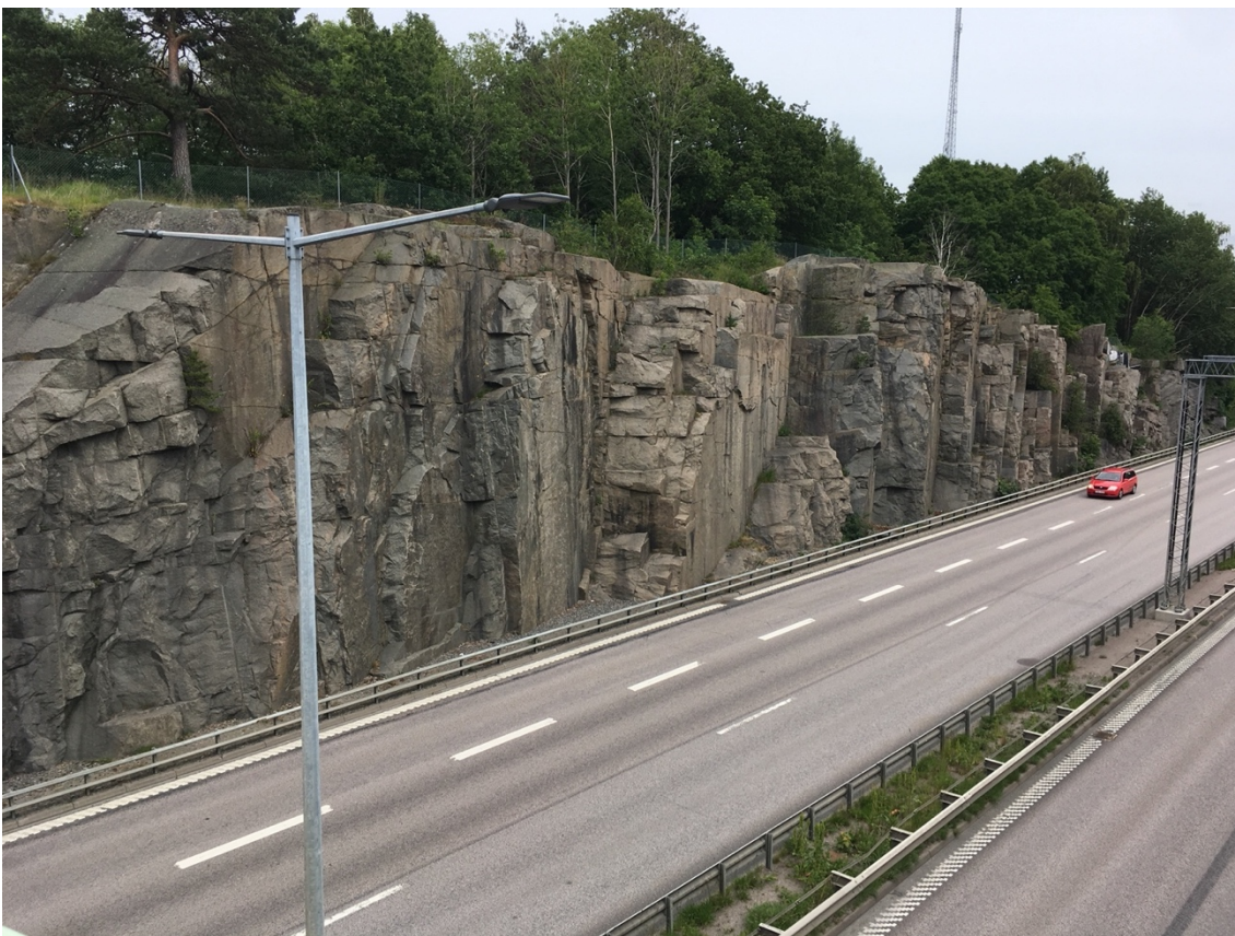
Figure 7. Vertical fractures in the road cut south of Västra Frölunda church. View to the east from the bridge.
