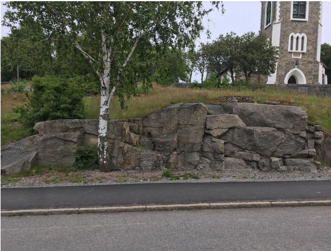
Figure 6. Vertical fractures at Västra Frölunda church, view to the east.
